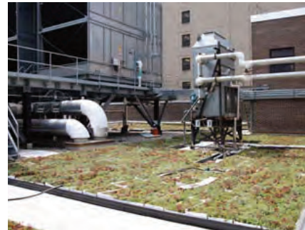
Green Roof - Data Center Rehab Fashion Institute of Technology
